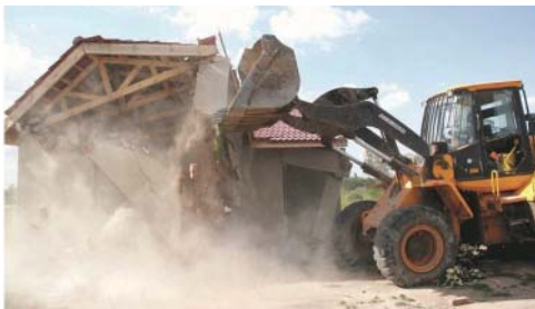
Figure 2: A bulldozer destroys an illegal/irregular house built on state land (Source: Sajeni 2021, in The DailyNews , 30 June)
